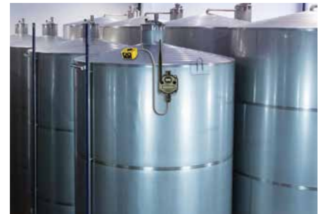
Tank Level Monitoring
